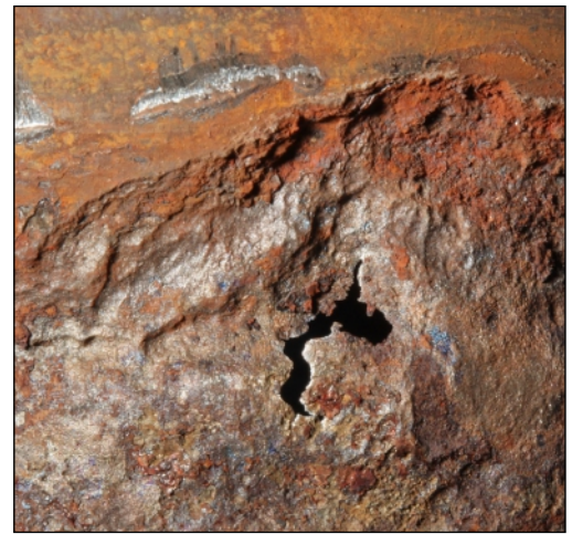
Corroded area of tube showing through-wall perforation.
