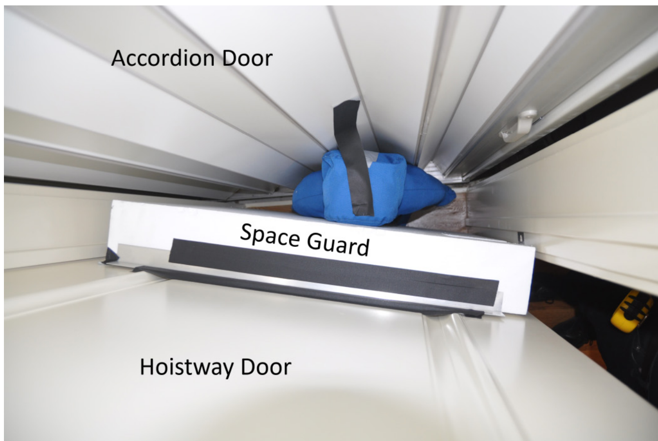
Figure 4. Retrofitted Space Guard with Blue Child Dummy
